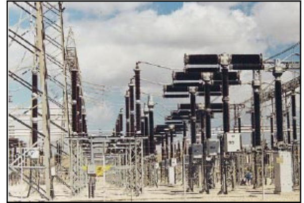
400 kV substation in Jordan
